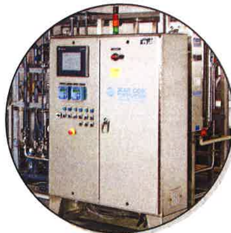
NEMA 4X control panel
